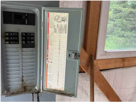
Main Panel, Detached Garage
