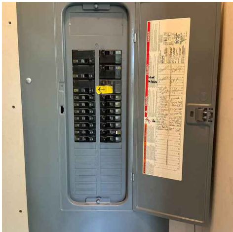
1st Floor North Subpanel
