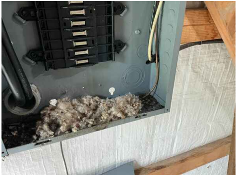
Main Panel, Detached Garage
