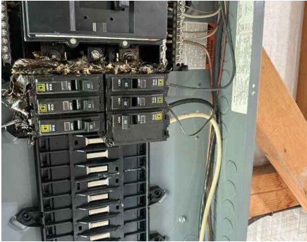
Main Panel, Detached Garage
