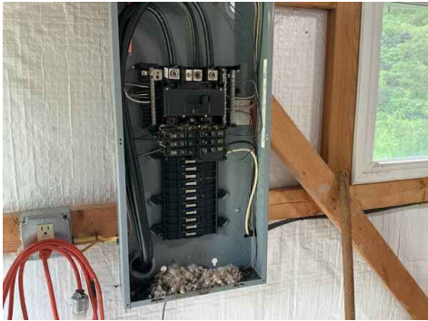
Main Panel, Detached Garage
