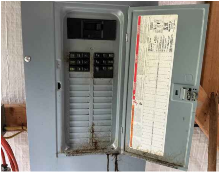
Main Panel, Detached Garage
