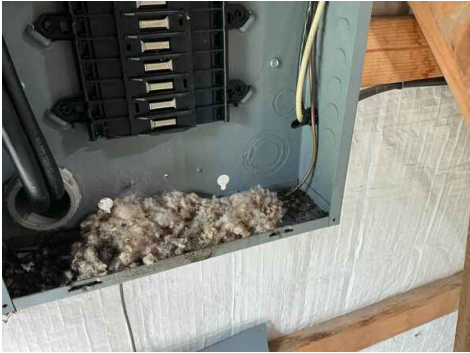
Main Panel, Detached Garage
